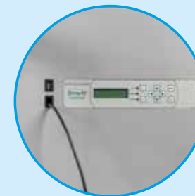
Control panel separated from robot for redundancy safety
